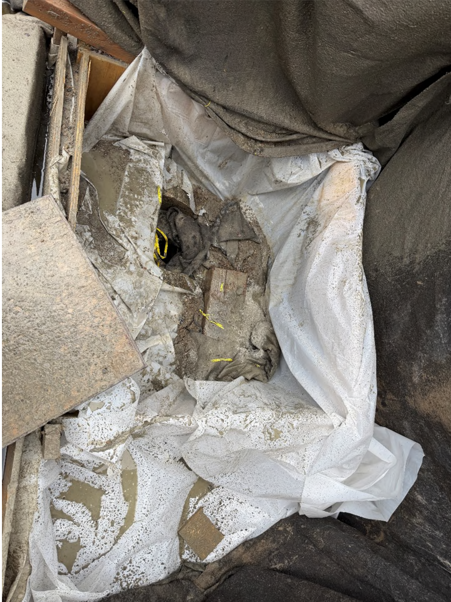
Debris enclosure around AH-2.
